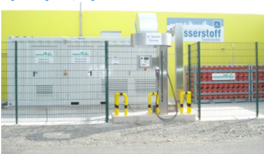
Figure 3.10: Hydrogen Fuelling Station, Cologne
