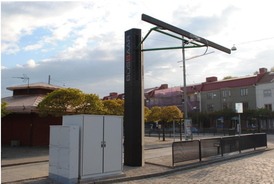
Figure 3.8: Overhead Charging Station for Plug-in Hybrid Bus, Gothenburg
