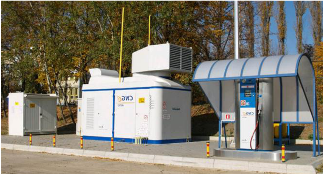
Figure 3.12: Typical CNG Fast Filling Station
